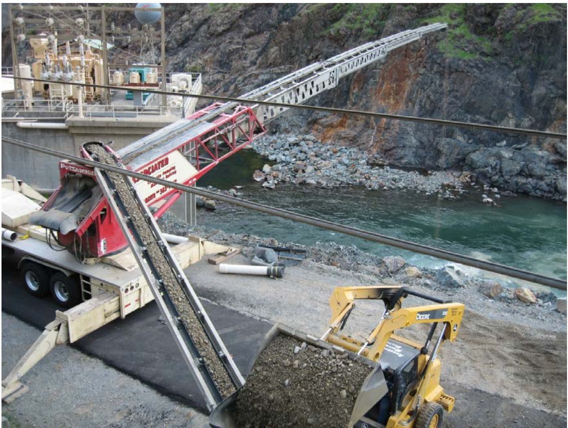
Figure 2.3. Gravel injection on November 29, 2007. Gravel pile is located in zone of aeration downstream of the Narrows II powerhouse.
